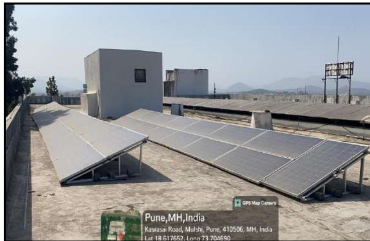
Photograph of Roof Top Solar PV Plant:
