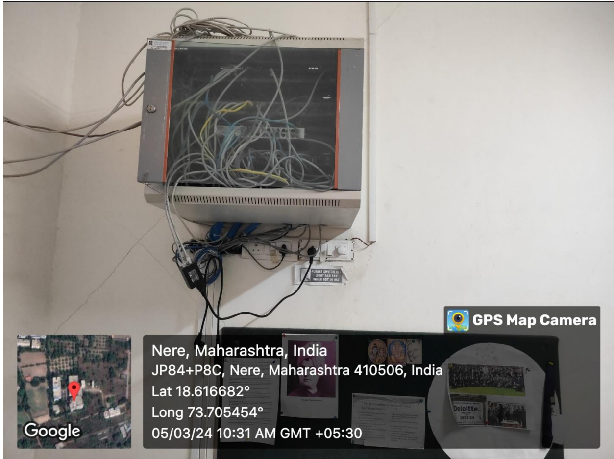
LAN Rack (Distribution Panel) for LAN connectivity in Institute premises
